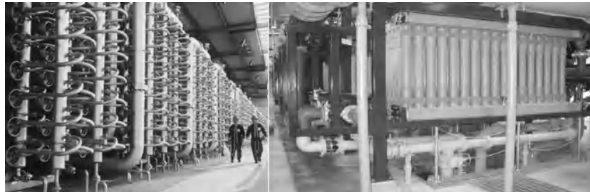
Figure 4.15. Industrial plant for desalination of seawater
